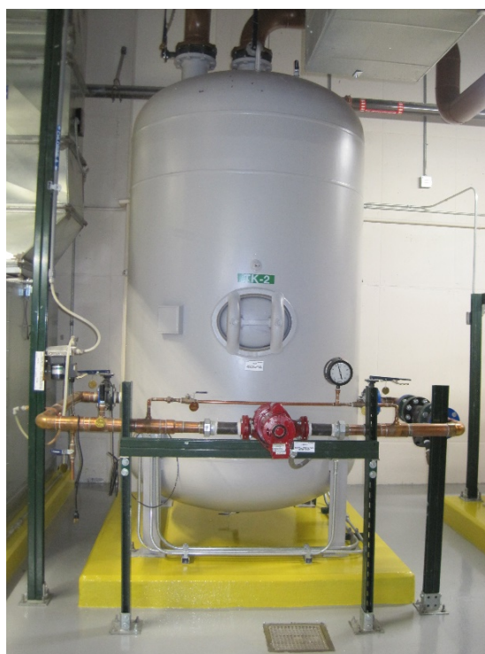
Photograph - NPDES-03A027-18-015 SCC Trinity Cooling Towers – Neutralization Tank
