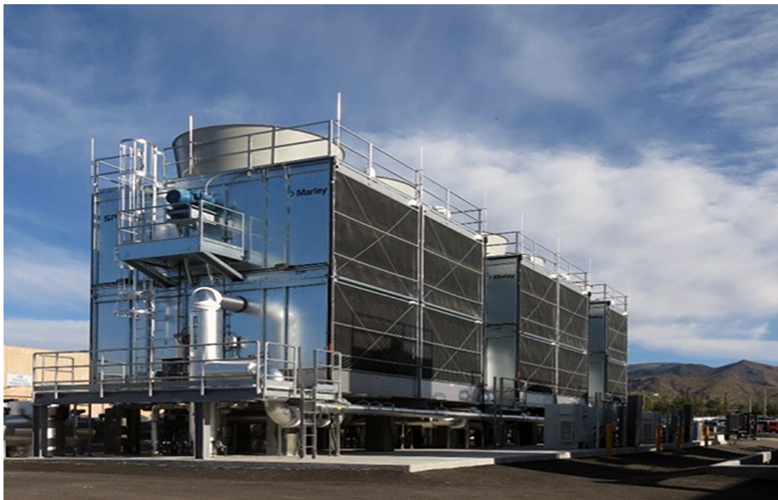
Photograph - NPDES-03A027-18-010 SCC Trinity Cooling Towers
