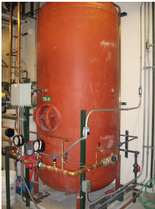
Photograph - NPDES-03A027-18-008 SCC Chiller Cooling Towers - Neutralization Tank
