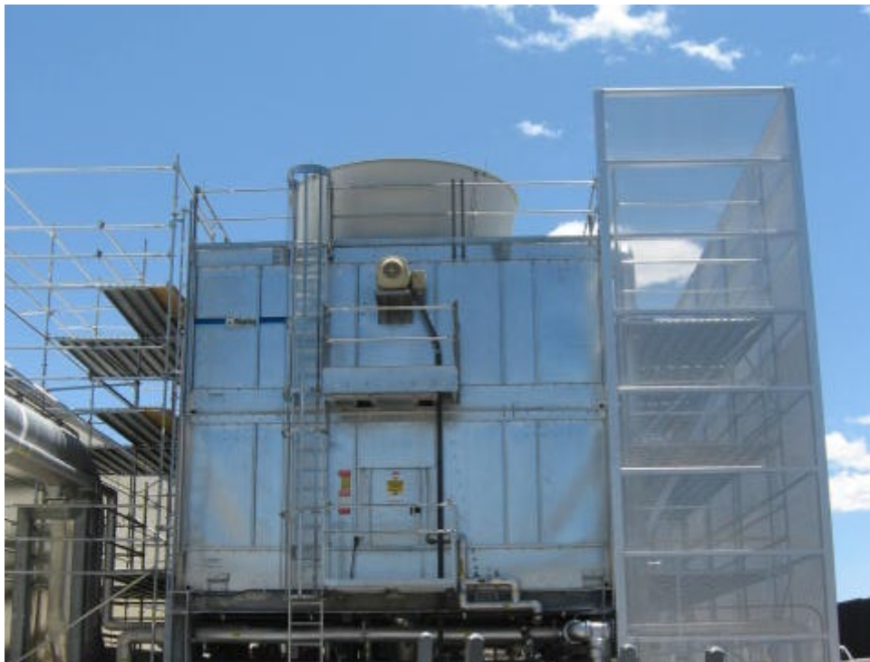
Photograph - NPDES-03A027-18-004 SCC Chiller Cooling Towers
