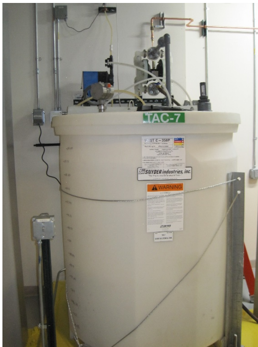
Photograph - NPDES-03A027-18-014 SCC Trinity Cooling Towers – Corrosion Inhibitor Feed Tank
