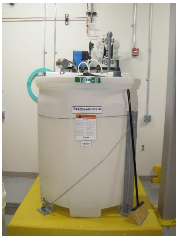
Photograph - NPDES-03A027-18-013 SCC Trinity Cooling Towers – pH Adjustment Chemical Feed Tank
