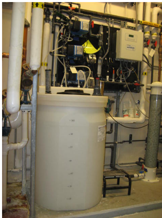
Photograph - NPDES-03A027-18-007 SCC Chiller Cooling Towers - Dechlorination Chemical Feed Tank
