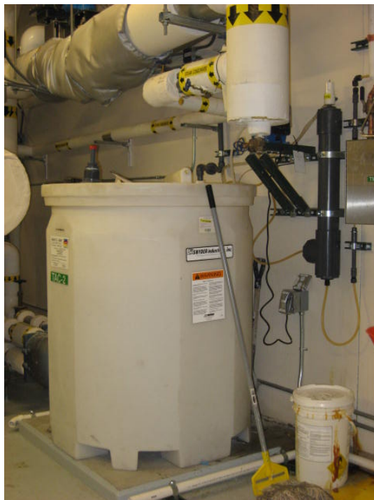
Photograph - NPDES-03A027-18-006 SCC Chiller Cooling Towers - Corrosion Inhibitor Feed Tank
