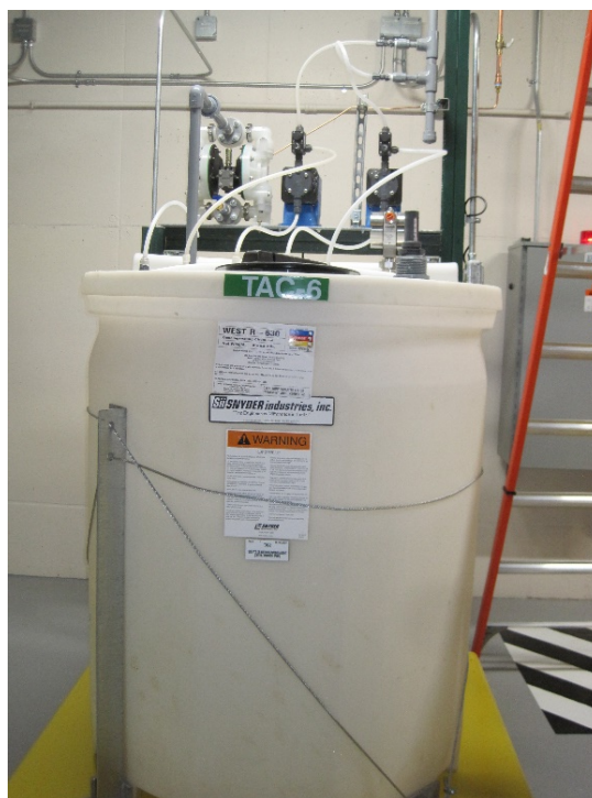
Photograph - NPDES-03A027-18-011 SCC Trinity Cooling Towers – Dechlorination Chemical Feed Tank
