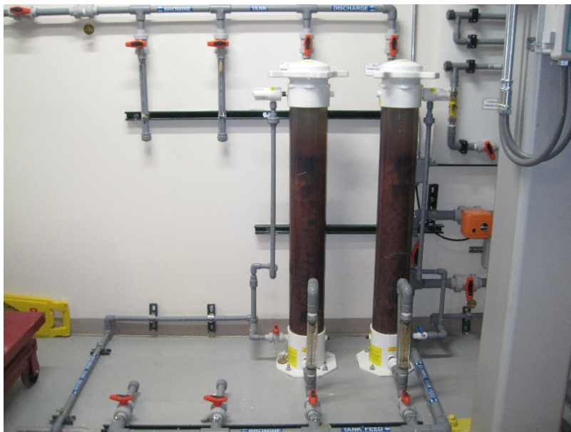
Photograph - NPDES-03A027-18-012 SCC Trinity Cooling Towers - Brominators
