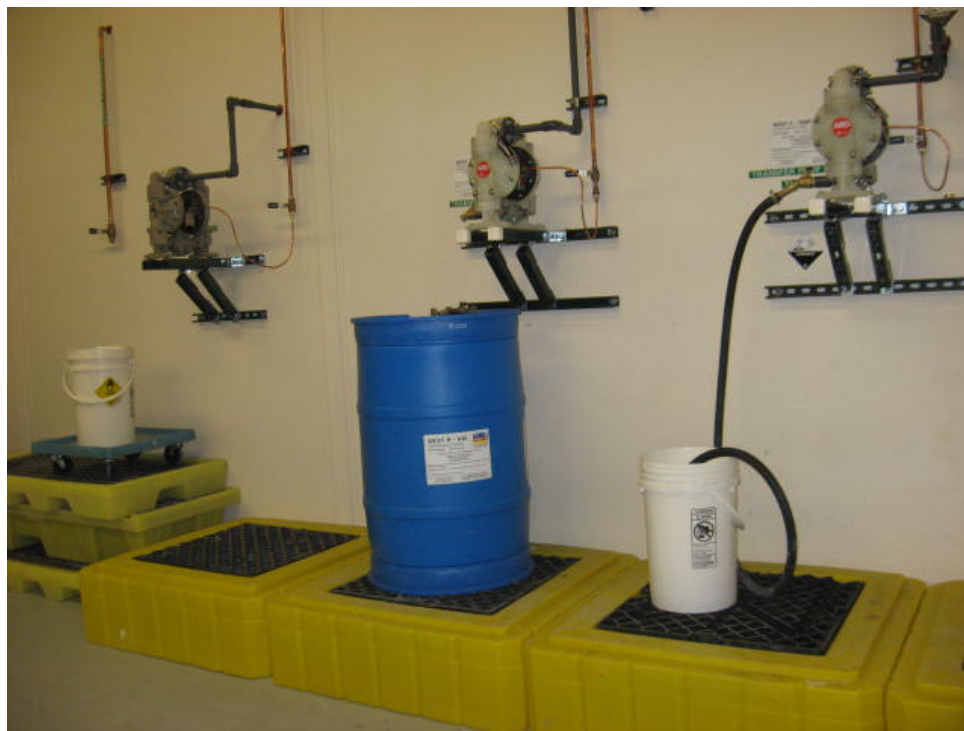
Photograph - NPDES-03A027-18-005 SCC Chiller Cooling Towers - Raw Chemical Feed
